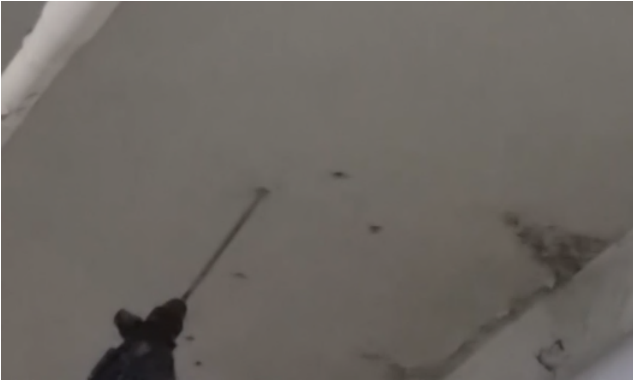
(1) Drill holes – check the cracks and drill holes to the rear side of the concrete structure, and clean the holes by air-compressor.
