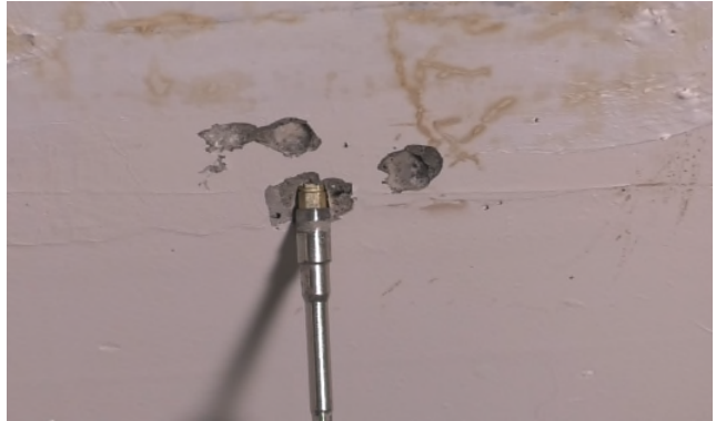
(2) Installing packers – insert packers into holes, and fasten packers tightly using T-wrench
